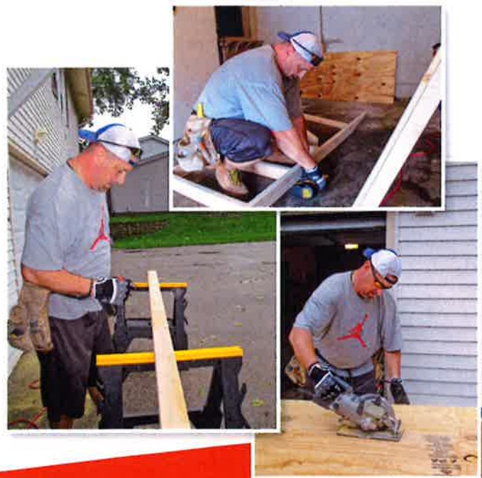
DuPage Senior Citizens Council Home Maintenance Program Ralph King building a ramp for a senior resident
